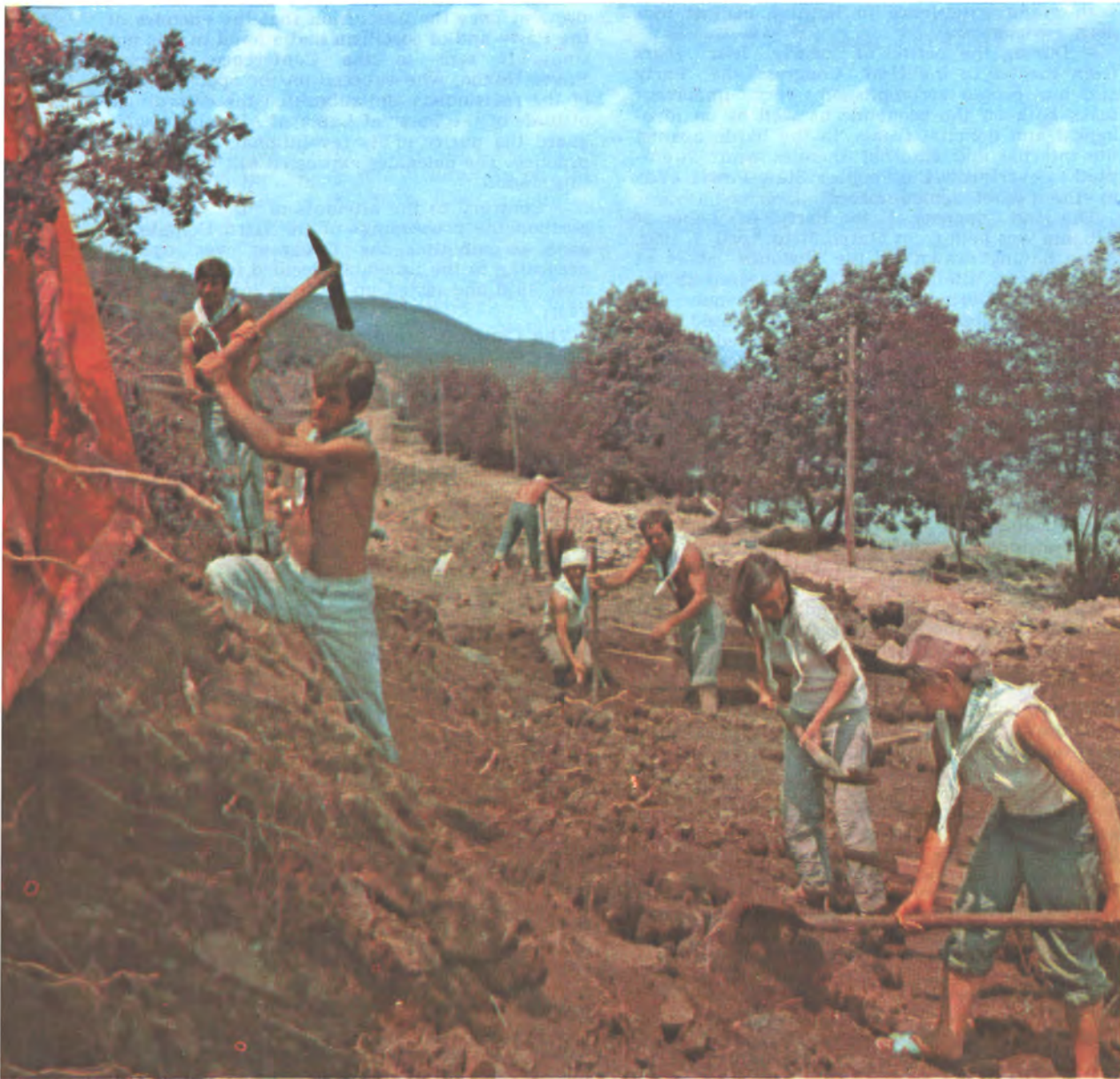
The new railroad track is continually extending through hills and rocky mountains.
