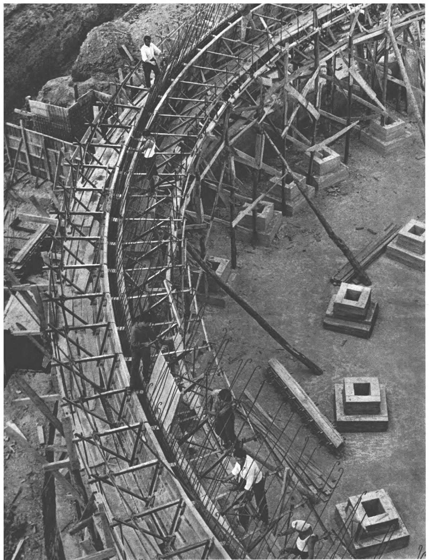
The work for the construction of the Fieri Urine Factory has entered a new important stage.
