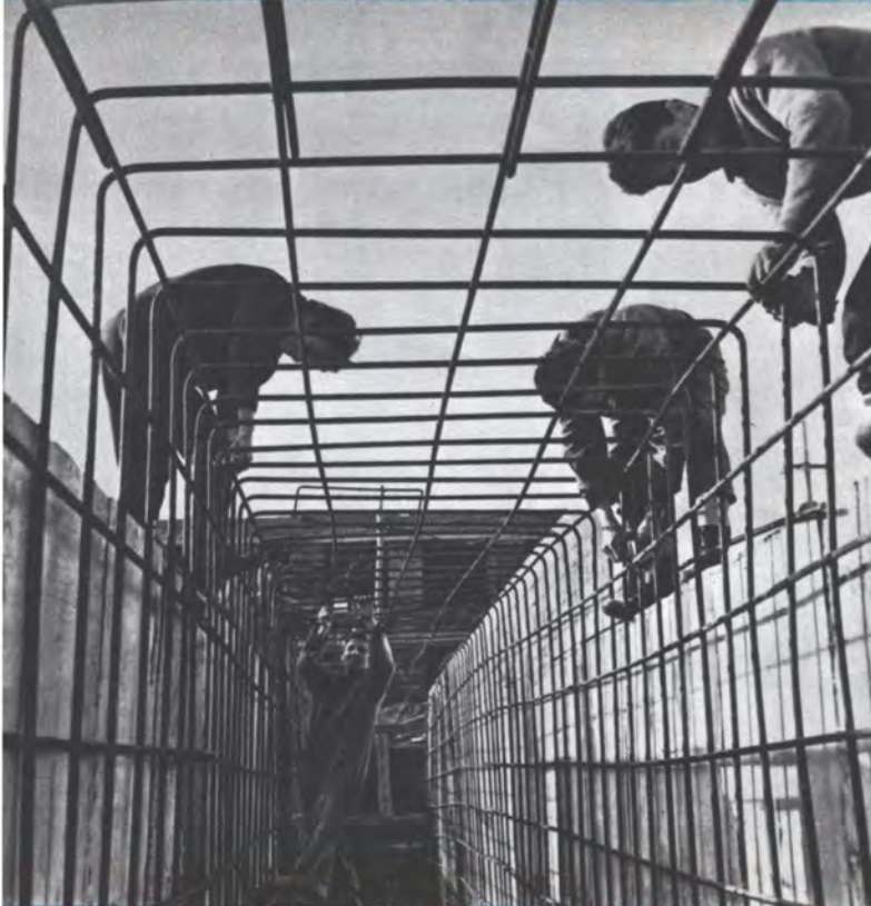
The first Nitrate-Enriched Fertilizer Plant in our country is being built in Fieri.
