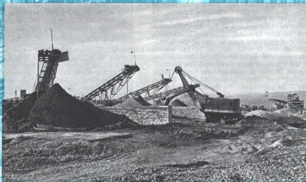
Partial view of the construction site of the Complex of Metallurgy in Elbasan.
